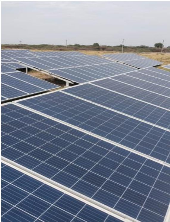
Captive Plant – 1.1MW
